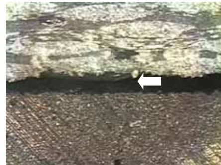
Fig.12 Debonding between carbon sheet and glass composites
